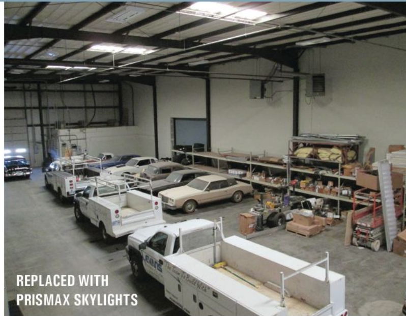
OLD TRANSLUCENT SKYLIGHT PANELS
