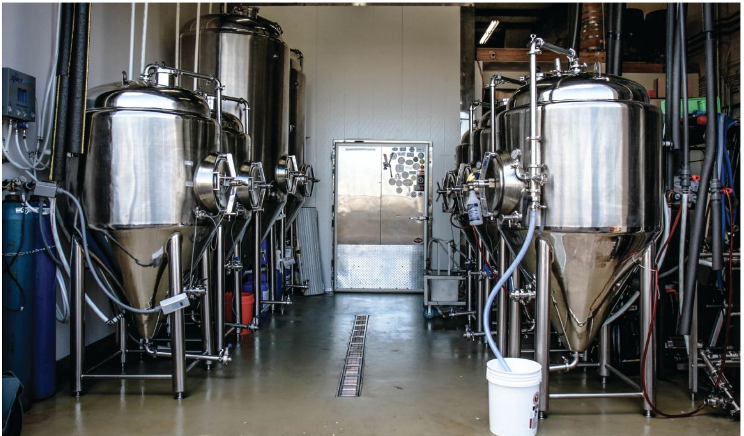
Above: Large fermenting equipment and glycol coolers require substantial space.
