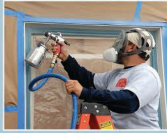
Facade Restoration – Field-Applied High Performance Coatings – Water-based Low-VOC Fluoropolymers – Anodized Aluminum Restoration
