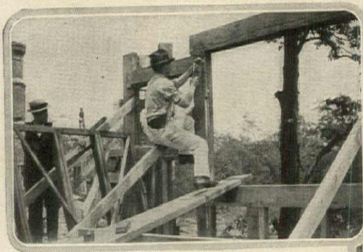
In this stage the first floor timbers are in place and the carpenter is cutting a groove into which to set the window frame
