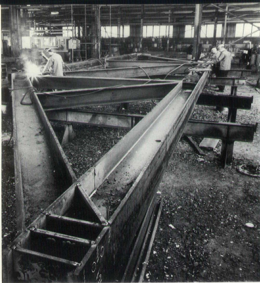
Huge 16-foot-deep welded trusses for the addition were fabricated in the Cambridge, Mass., shop of A. O. Wilson Structural Company. Upper floors three through six in the addition will be "hung" from a main grid of the deep interconnecting trusses, most of which will span the building's nine basic 58-foot module areas. Sloping steel-framed roof of the new library structure will also be supported by the trusses (note angled structural truss member at left).
