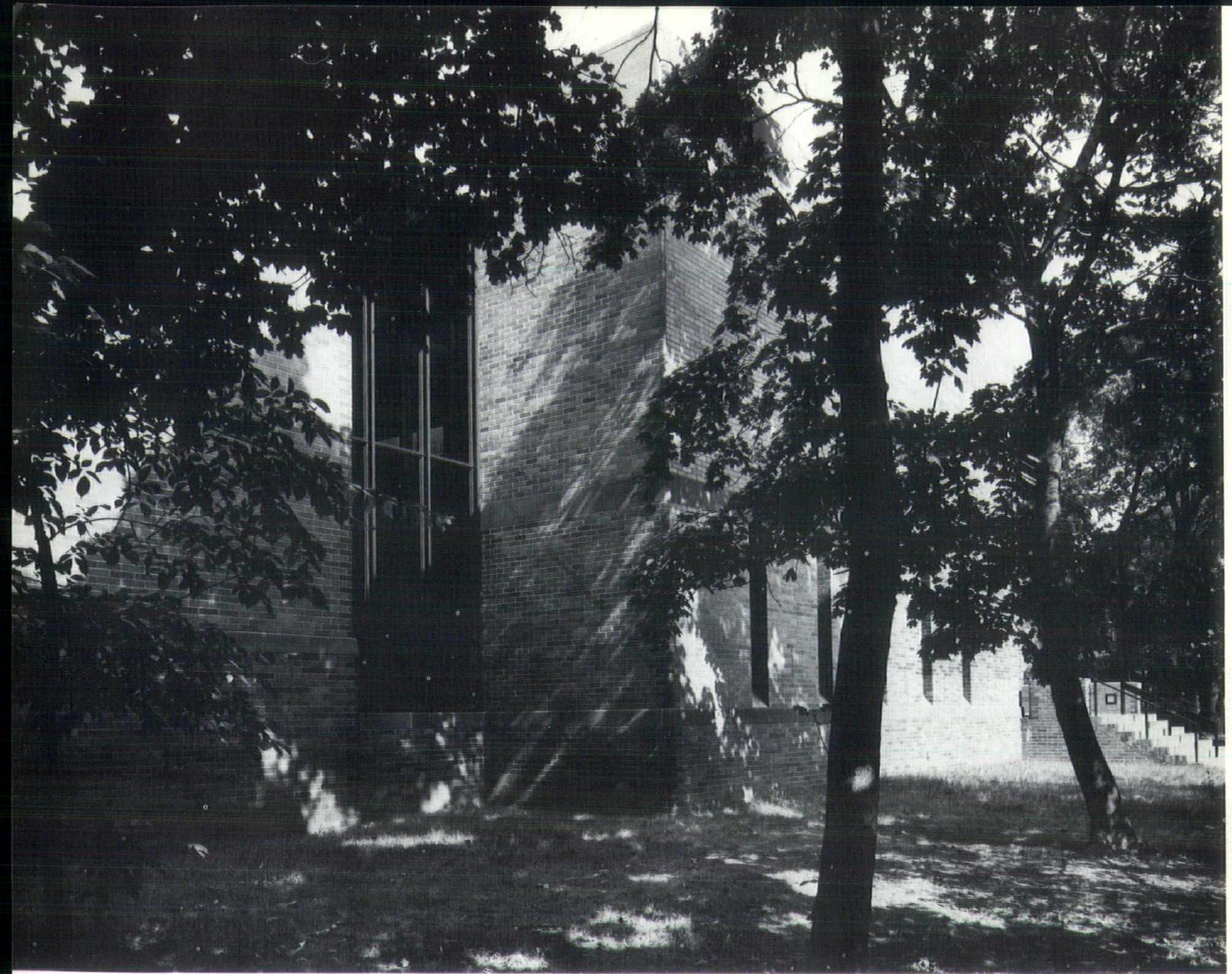
The new building has masonry bearing walls. The smaller spaces are spanned with bar joists, while the large space has a roof structure of precast concrete Tees.
