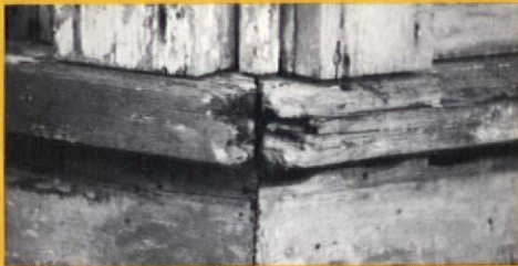
This rotted - and irreplaceable - woodwork...
