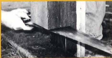
10" rotted bottoms of these load-bearing columns...
