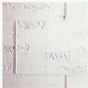
Even before paint, groups of cavities divided into blocks by thin mortar joints effectively create Travertine texture.
