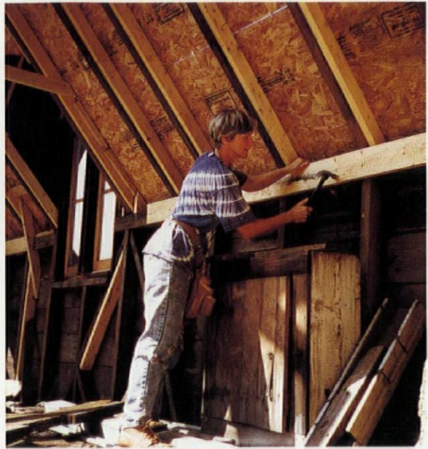
With a solid floor underfoot and a sound roof overhead, Sharon finishes up on the interior.
