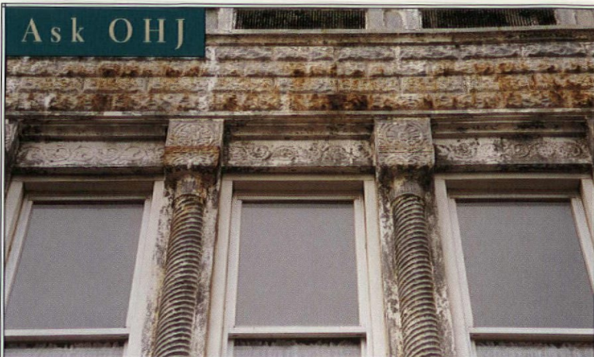
Left unpainted, this prefabricated steel façade is vulnerable to rust.
