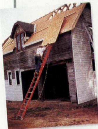
After we installed new sheathing and shingles, the building was dry for the first time in decades.
