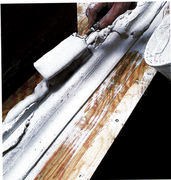
Above: By the fifth and sixth runs, Frank is troweling in a much thinner plaster mix to build up the profile. It doesn't stay liquid long, however, as the curing moulding accelerates the setting time of the fresh plaster.
