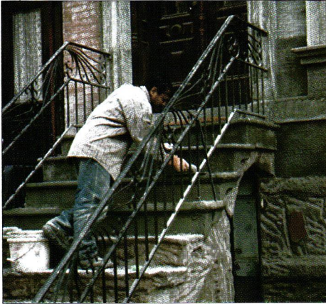
A mason applies patching material to the front steps of the Fort Green brownstone. Note the scratch marks in the stone.
