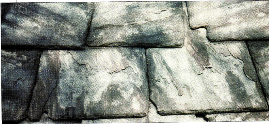
This Pennsylvania Hard-Vein slate has reached the end of its serviceable life. Note the numerous cracks, indicating loss of strength, and the severe delamination that allows the slate to absorb moisture.
