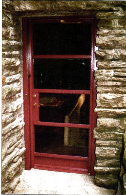
Left: The Conservancy feared that the bridge entrance (in effect, a large steel window) would have to be replaced, but patching allowed the crew to retain nearly all the original parts. Below: Bob Seekircher brazes replacement steel into the door frame.
