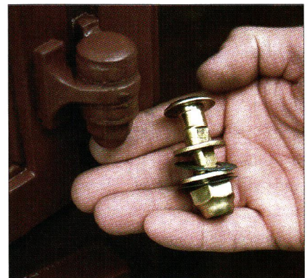
Top: Surface rust on the door frame is typical for most of the building. Middle: Finger catches on the corner windows have one moving part. Above: The oversized barrel hinges pivot on large bolts, which were removed and cleaned to free up several windows. Nuts and washers are adjusted for just enough friction to hold the window open in a breeze.
