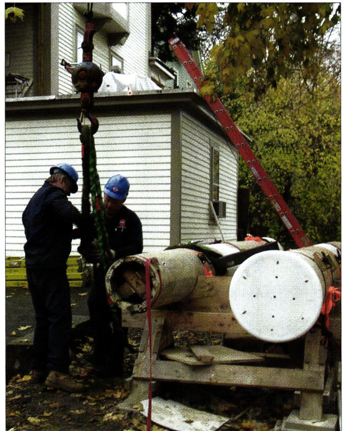
The columns, waiting for reinstallation, show a rebuilt bottom with vent holes, next to a top, still in good condition.
