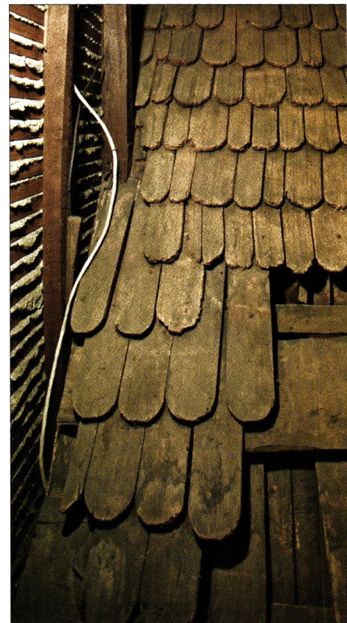
The 18th-century addition was built over the existing roof, preserving its wooden fishscale shingles, which can still be seen from an attic space on the second floor.
