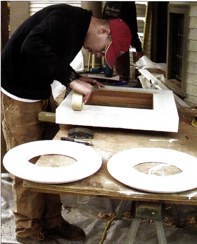
Decay below the column shafts was extensive. The plinths and bases had to be completely rebuilt out of mahogany.
