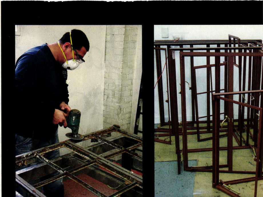
ABOVE: Omar Hernandez works to strip a vintage Hope's casement window down to bare steel. The windows, with steel muntins removed, have been primed and are ready for the installation of the smaller-paned glass inserts with lead caming. (Original muntins are saved and used on other jobs.)
