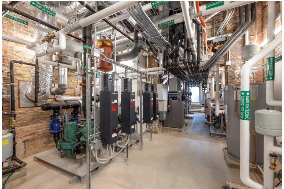
Behind its 165-year-old walls, the building now operates with modern efficiency, powered by a state-of-the-art geothermal system.
