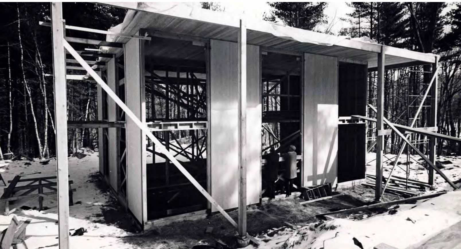
System House, historic view of house during construction, ca. 1961 (photographer: Syd Greenberg, source: New Canaan Historical Society)
