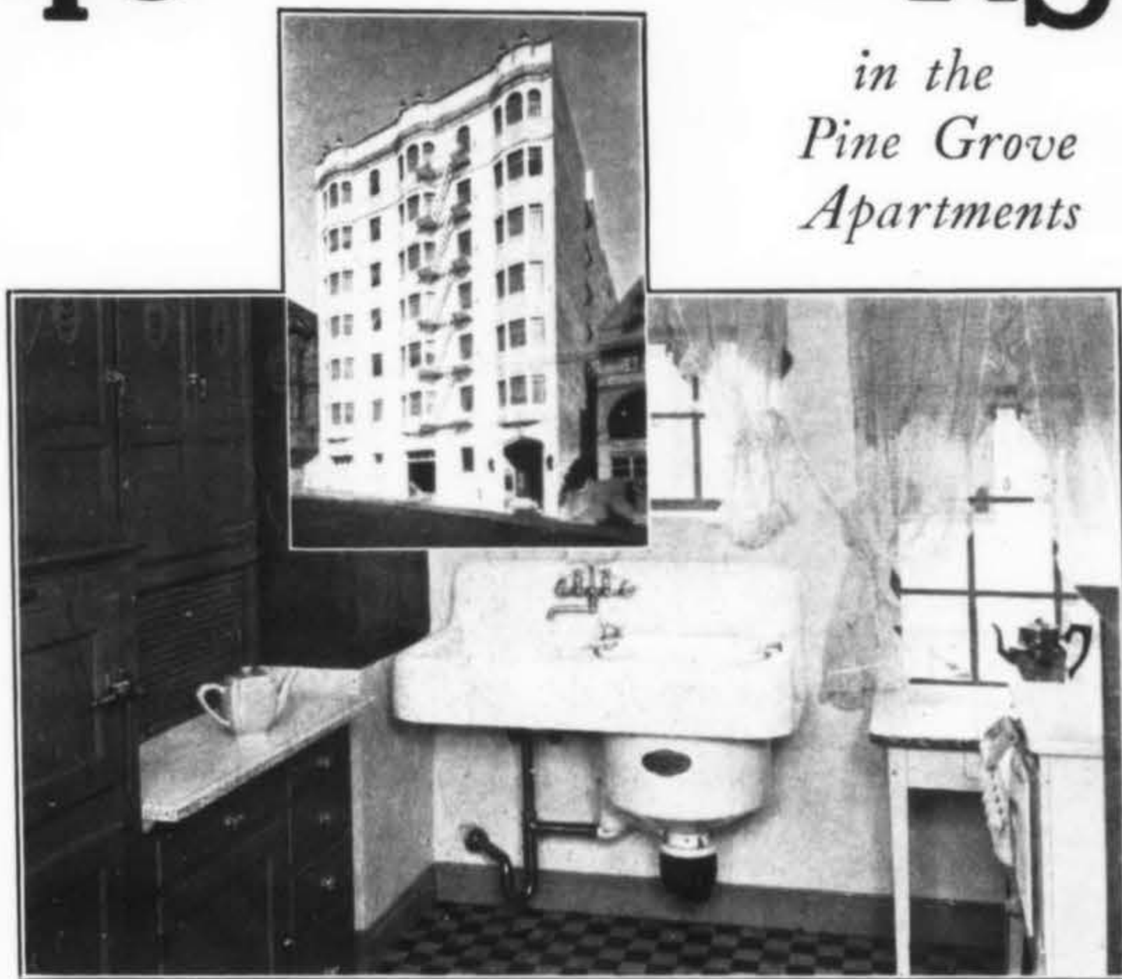
WALKER Electric Dishwasher Sink, Model 114-R, installed in the kitchens of the Pine-Grove Apartments, San Francisco.
