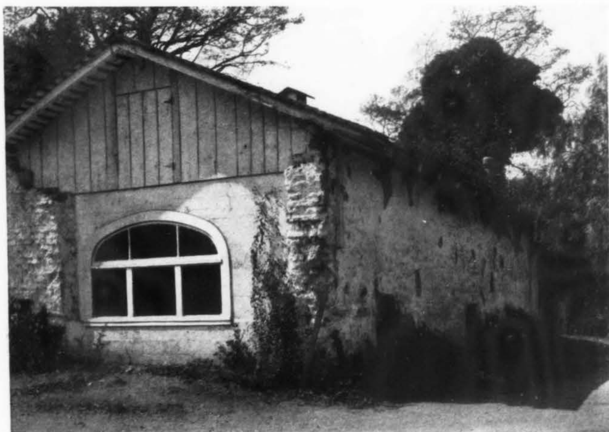
A closer view of the ball room; the concrete end wall is recent
