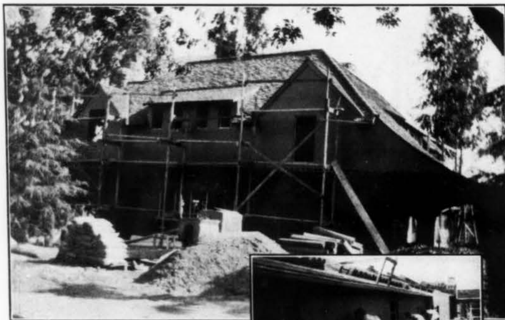
The residence illustrated above on North Rexford Drive, Los Angeles, was built by E. A. Kaiser. The plastering was handled by Kurbishley & Lane. Sisalkraft was used back of the stucco.
