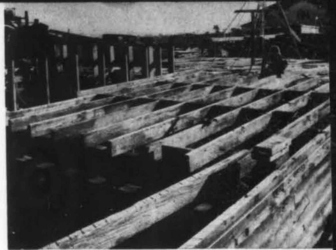
Pressure treated lumber for home of Dr. John L. Pomeroy at Brentwood being placed.
