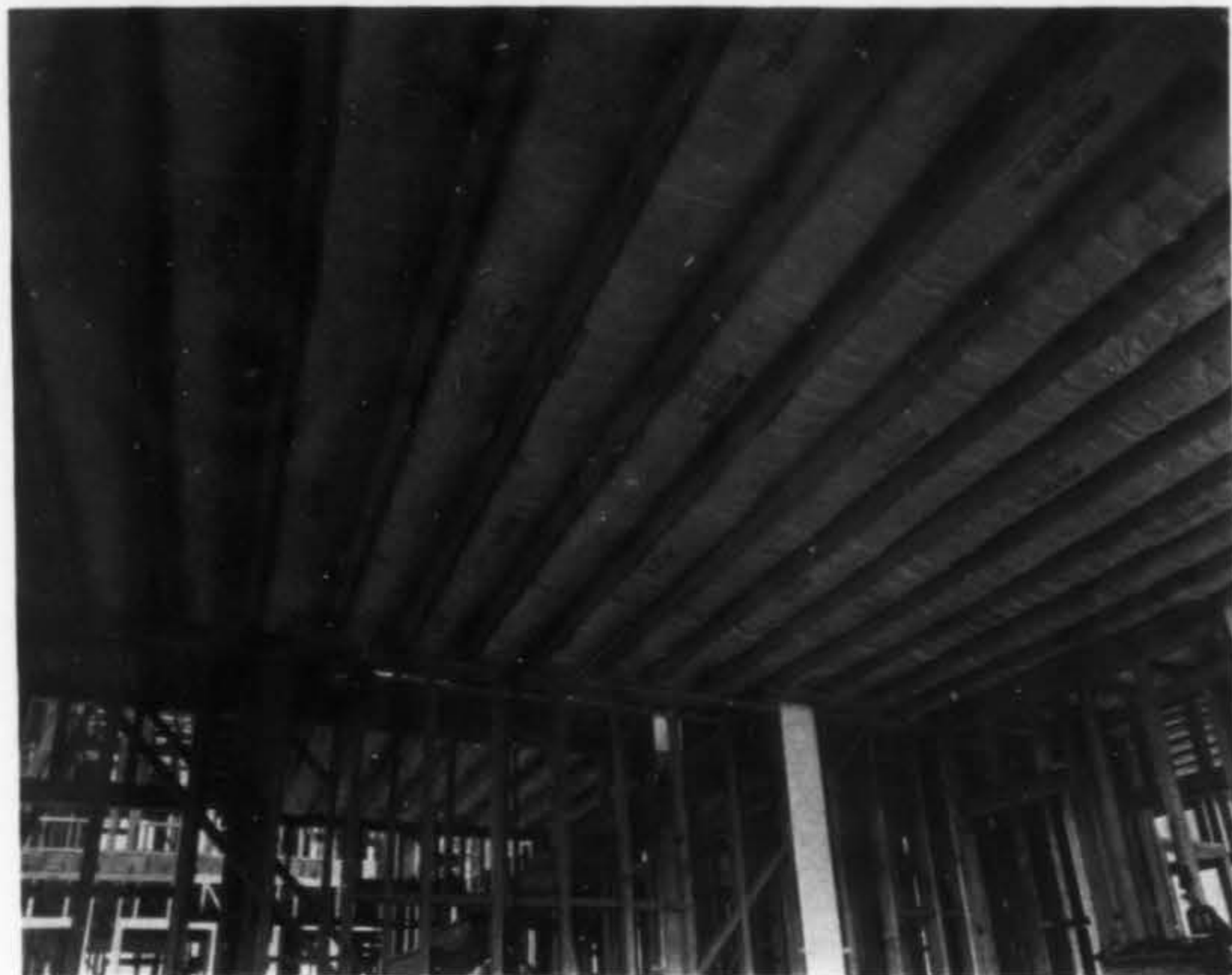
This most efficient method of ALLTITE soundproofing for floors as well as PAK-FELT under roof for heat insulation was selected in the Howard Hawks residence.
