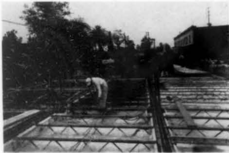
Above: Floor system showing special technique. Below: Gypsum tile used in walls.
