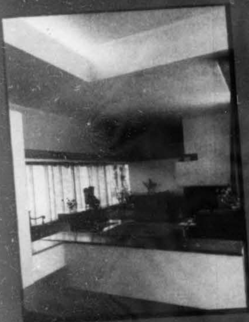
In the living-dining room the warm air register is an inconspicuous part of a stainless steel grille above the windows. Cold air returns are provided at floor level.
