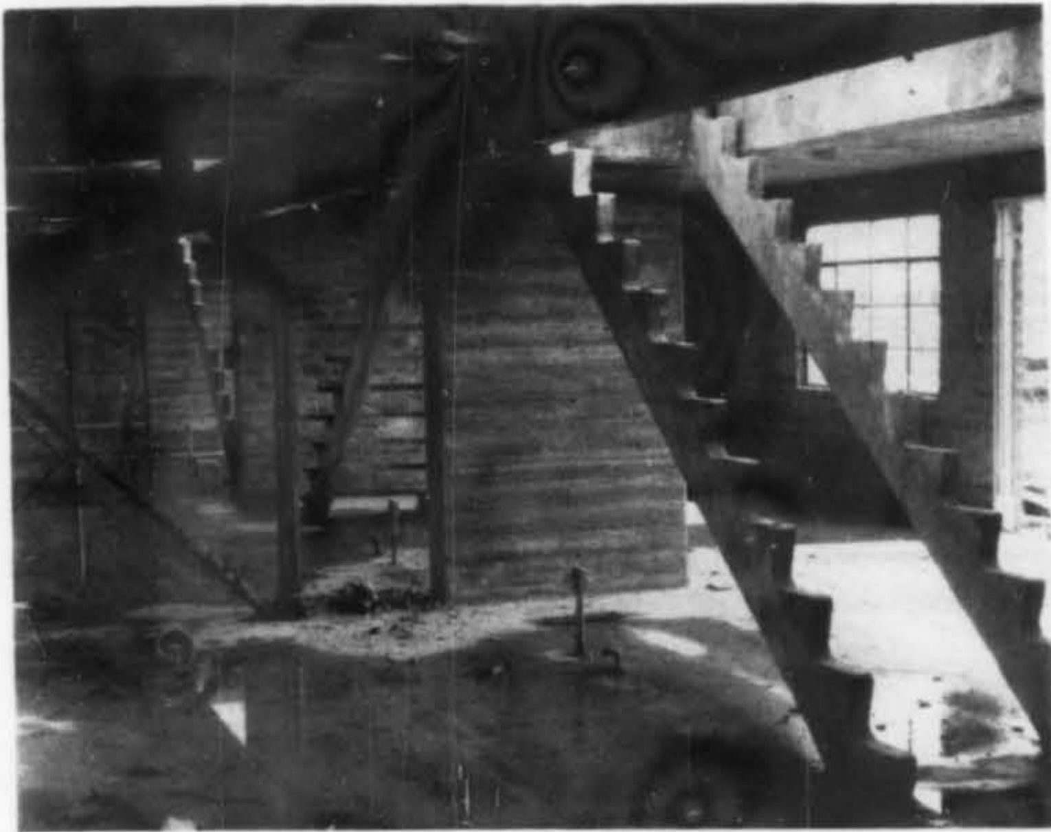
A CONSTRUCTION VIEW OF THE LOWER FLOOR OF ONE OF THE LIVING UNITS
