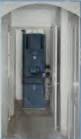
Each Furnace Is Installed in a Closet.
