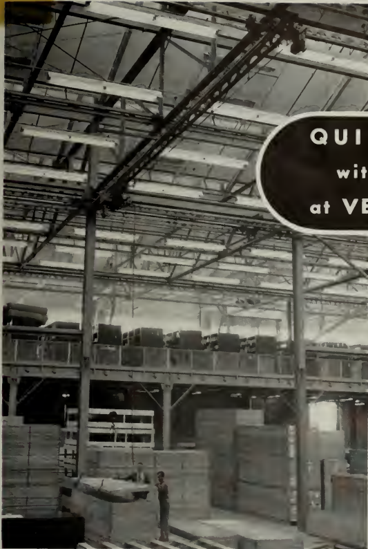
Cleveland Tramrail crane serving new warehouse building at Vega. Hoist, trolley and bridge motions are motorized and controlled by convenient push-button station.
