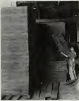
Therman ready to be installed at the Douglas Aircraft Company plant at Long Beach. Approximately 2,000,000 sq. ft. are being used.
