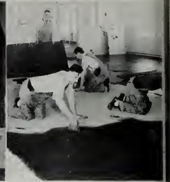
Below: The interior walls of the Henry Hoover School, Whittier, were formed against Plyform. There was no plastering. Paint was applied directly to concrete.
