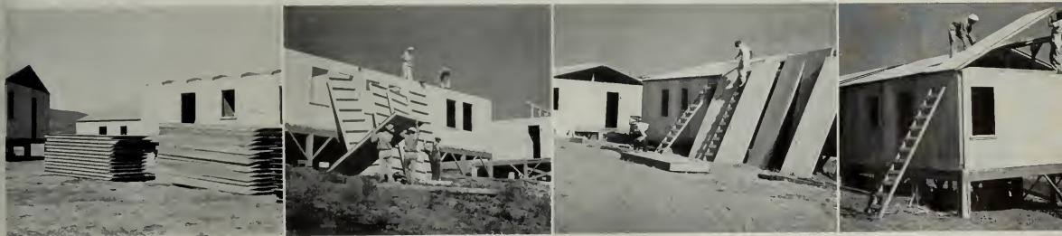
The use of plywood structures for national defense housing makes possible great speed in execution without sacrifice of structural strength. Below: Prefabricated roof sections are put into place for final completion.
