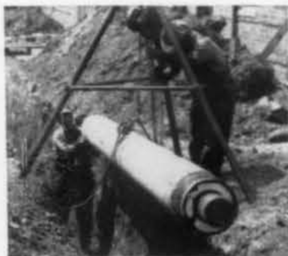
Section of Ric-wil prefabricated insulated steam conduit being lowered into shallow trench for steam connection to a new apartment at Shaker Square.
