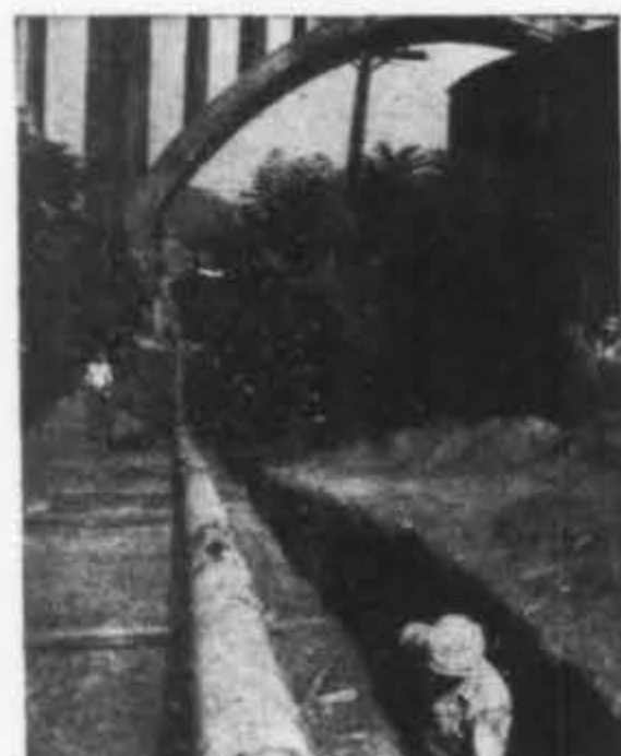
Welded into a single piece 700 feet long, this pipe was lowered into the shallow trench beside it, a section of the 2000 foot connection to the city main.
