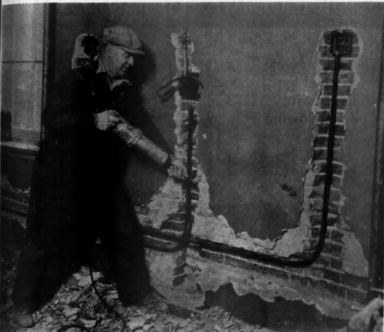
Workman Armed with Electric Hammer Cuts Out Chases for Pipes in About One-Tenth the Time Doing It the Old Way.
