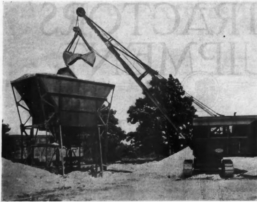
A \frac{3}{4} -Cubic Yard Clamshell Crane Charging Bins for Low-Cost Concrete Work.
