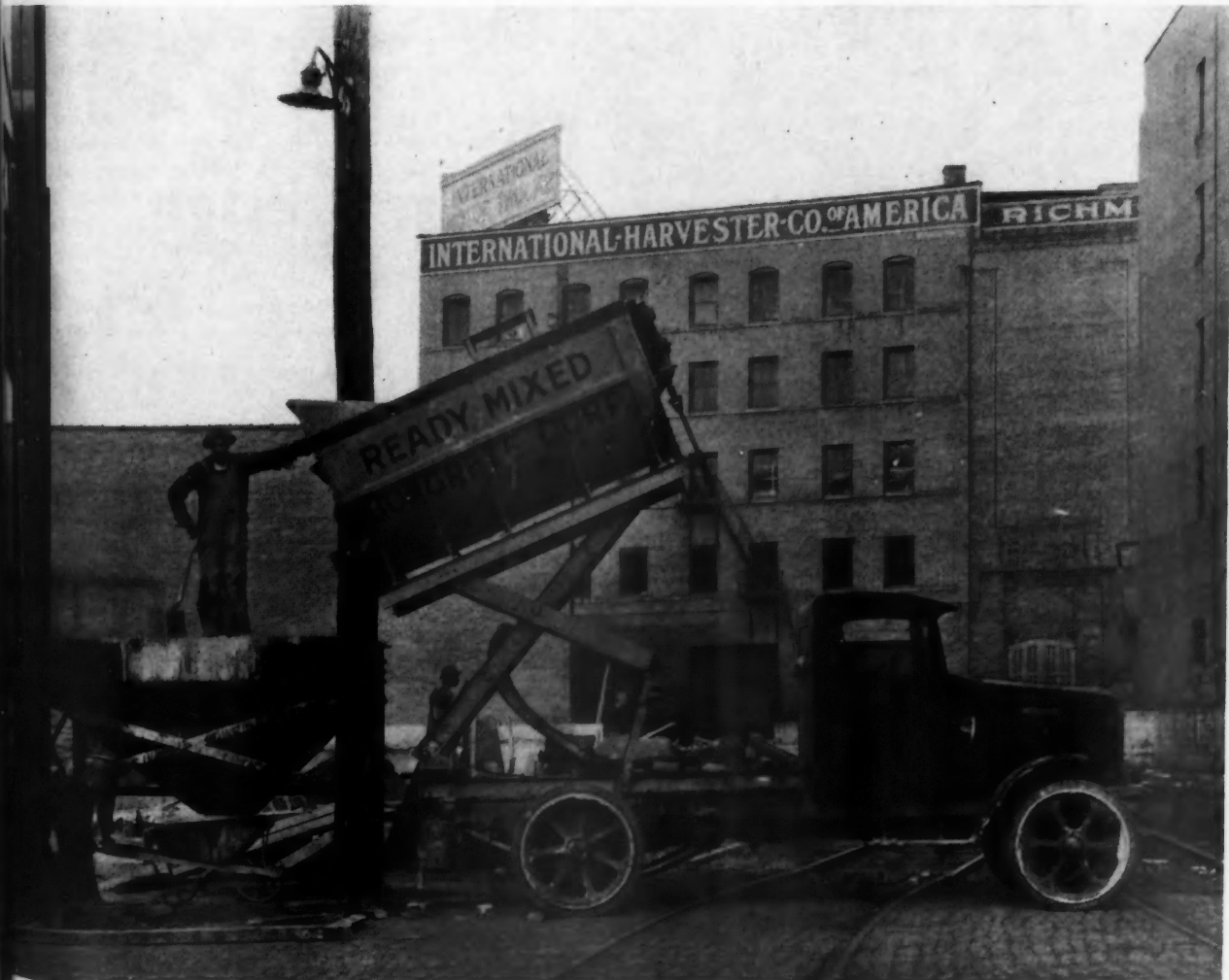
Many Cities Builders Are Now Buying Their Concrete Already Mixed, from a Central Mixing Plant. This motor truck mounted equipment delivers the mixed concrete to the job.
