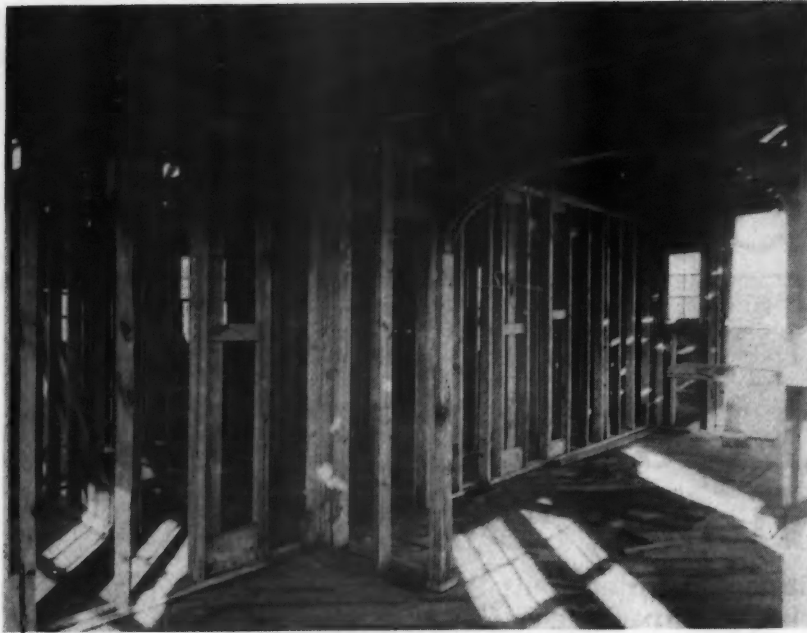
The Tenth Day of Construction with the House Fully Enclosed and the Work Progressing According to Schedule Laid Down by Roth Brothers, Inc.
