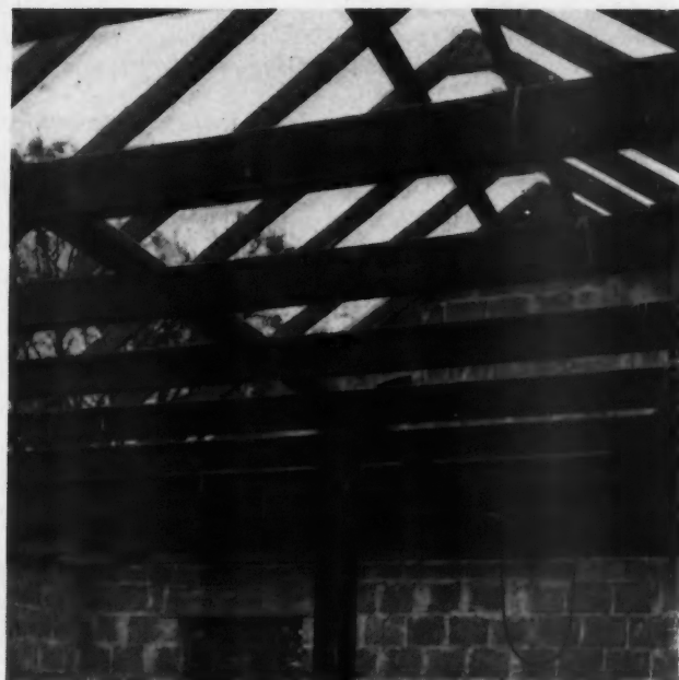
Here May Be Seen the Steel Construction of the Second Floor Ceiling and the Roof. A two-inch sub-roof of concrete was placed on the steel rafters.
