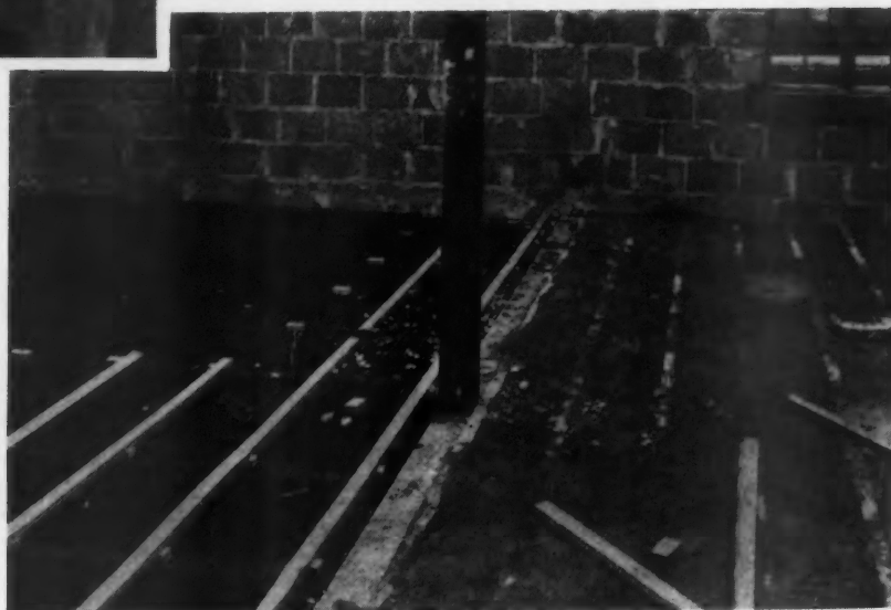
This Shows How the Concrete Floors Were Laid Over the Metal Lath with Sleepers Imbedded for Nailing Down the Hardwood Floors.
