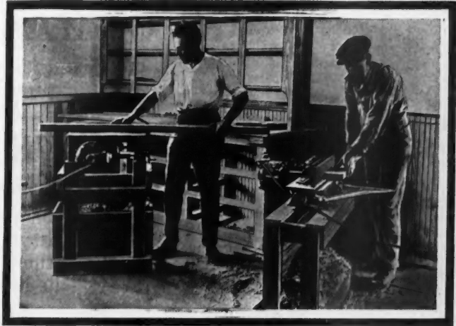
This photograph shows how one contractor saves money by applying "The Wallace Idea" to his business. C. B. Lynde, Jr., of Clinton, Mass., does his own mill work right on the job. Wallace Portable Machines double the amount of work done by his men and greatly increases his profits on each job.
