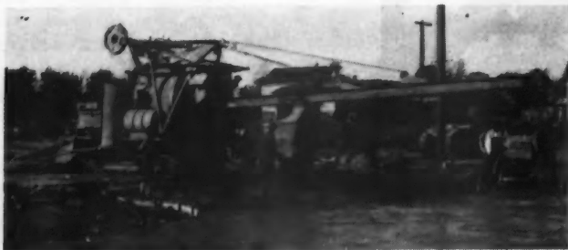
This Paver Is Now Equipped with an Automatic Control Which Relieves the Operator of Over 2,000 Hand Operations Daily.
