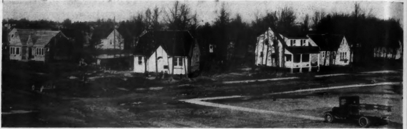
This View Shows a Group of Roth Homes Under Construction. It is a part of the construction undertaken for the Modern Housing Corporation and must measure up to the standards of that organization as well as to the high standards set by Roth Brothers, Inc.
