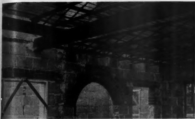
Looking Up at the Steel Construction of the Second Floor. Note how the steel beams are fitted into the bearing walls of hollow concrete tile.
