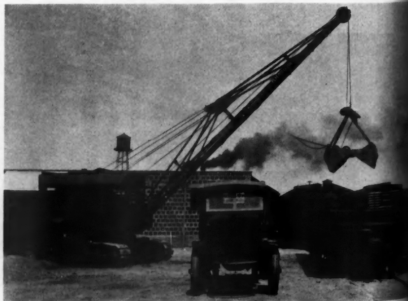
Clamshell Crane in the Modern Material Storage Yards of Baker & Holmes Jacksonville, Fla.
