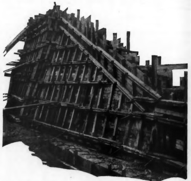
Reinforced Concrete Construction Work of All Kinds Is Greatly Simplified by the Use of Form Clamps Such as Are Being Employed on This Job.
