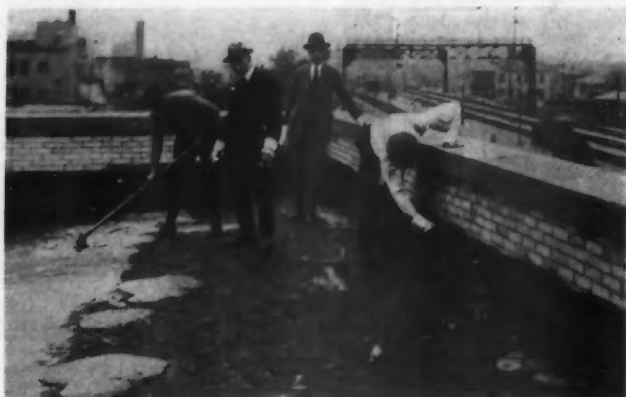
Malleable Asphalt Being Applied on Roof and as Side Wall Flashing on Union Station, Joliet, Ill., Fall of 1925.
