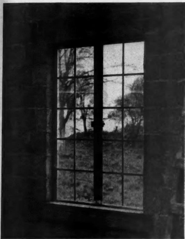
The Steel Casement Windows Were Fitted Into Grooved Tile and Sealed with Mortar.
