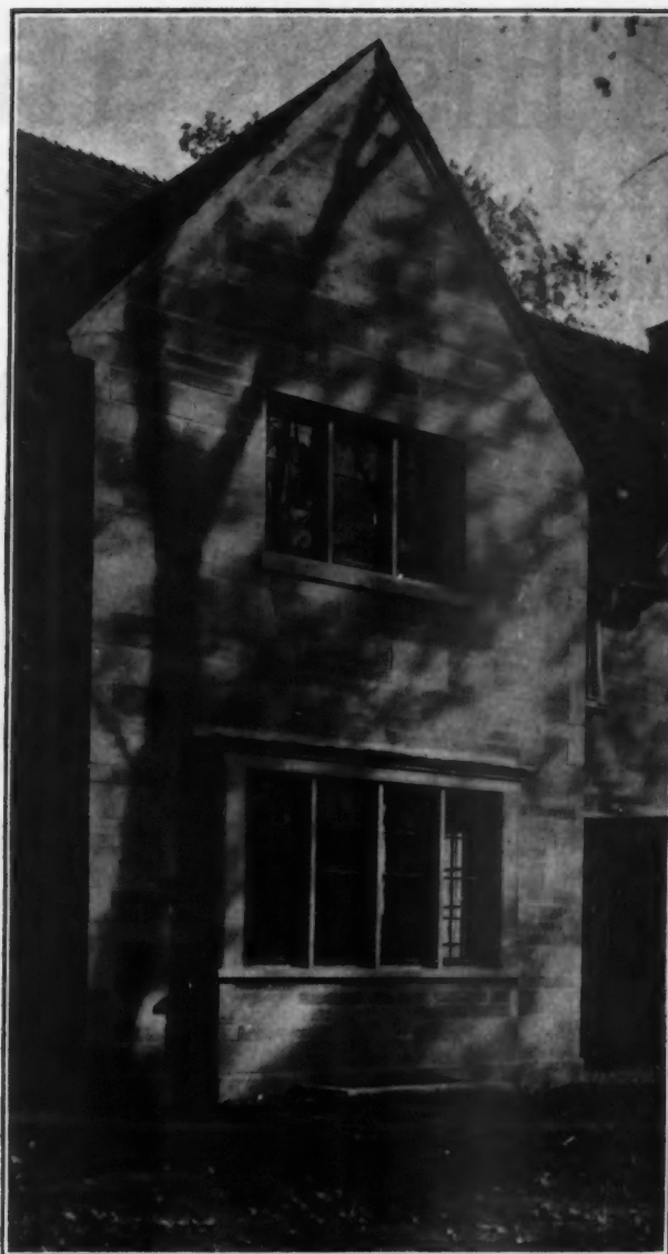
This detail view shows one of the common schemes for laying up the Random Ashlar class of Indiana Limestone.
