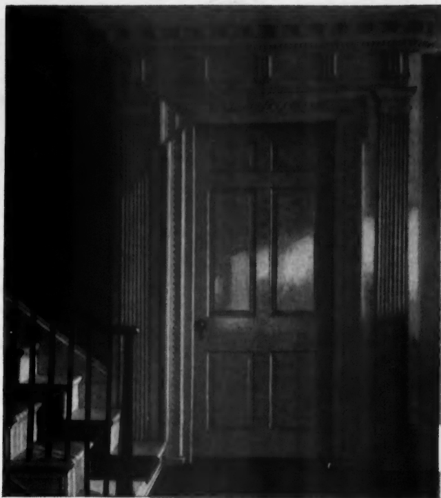
Detail of Pine woodwork on first floor hall doorway of the Cowles-Lewis House, built about 1760 at Farmington, Conn. (From White Pine Series of Architectural Monographs)
