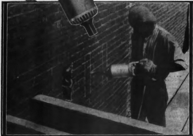
This laborer with a Syntron Hammer cut 67 Jolt Holes in a shale brick wall in one day. Average, 55 per day, saving $572 and 8 days' time.
