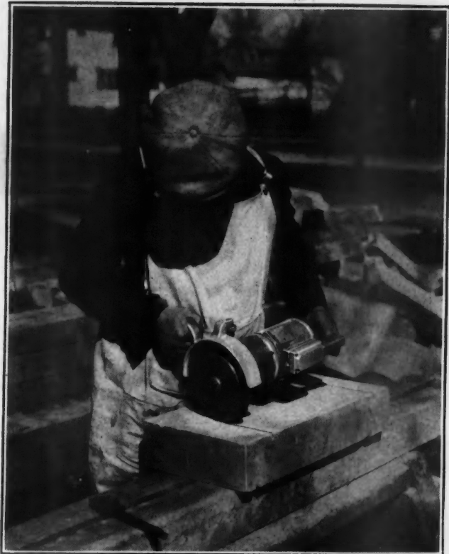
Electric saw replaces old-time mallet and chisel for breaking Indiana Limestone. One man now keeps six stone masons busy!
