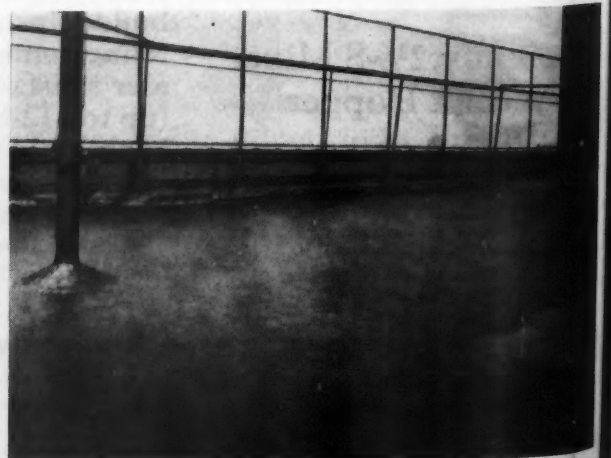
After the Mastic Is Applied a Permanent Repair Has Been Made as It Will Adhere Perfectly to Any Solid Surface.
