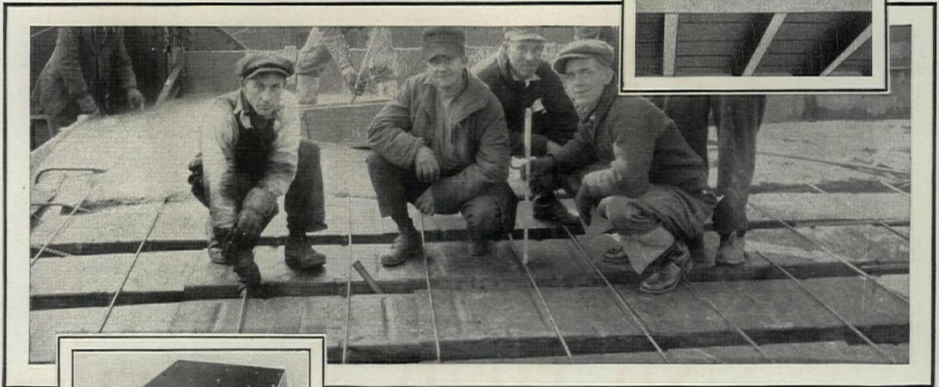
Note the rigidity of Meyer Steelforms. The heavy 16-gauge sheet steel permits walking and trucking over the forms without bending them. This speeds up work on the job.
