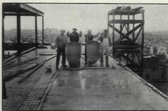
Nearing completion. The concrete is poured on the reinforcing fabric without requiring forms or props.
