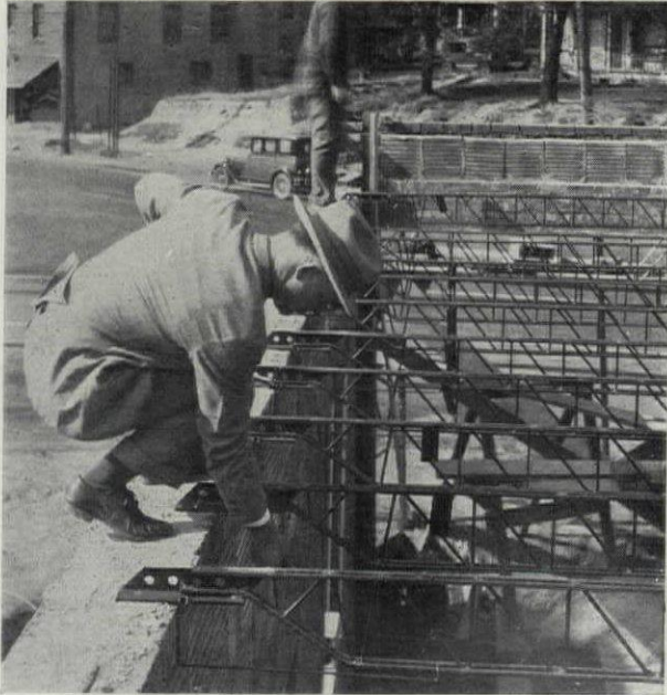
Most Open Web Type Joists Use a Ceiling Bracket to Extend Lower Chord to Wall for Ceiling Lath
