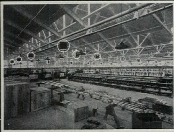
Thermodine Unit Heaters in one of the large eastern silk mills.
