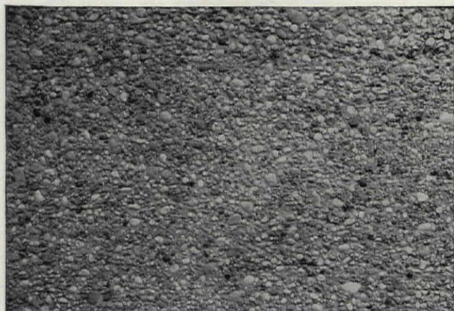
THE BOND EVERLASTING— Detail of Full Rough Area of Clean Stone on Concrete Exposed for Bond by Bonding Con-Text
