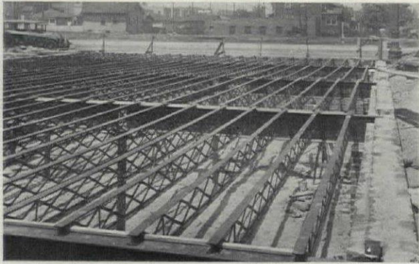
Rolled I-Beam Section With the Web Slotted and Expanded Into a Lattice Truss
