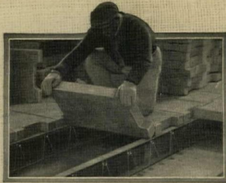
From actual photographs of the Henry Rachlin Apartment building at East Orange, New Jersey. Floor and ceiling constructed of Pyrobar Interlocking Structural Tile
