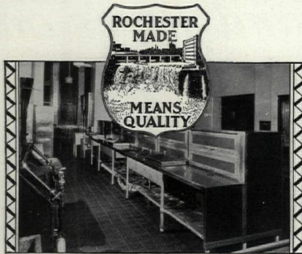
All-Monel Metal service counter in service kitchen of Rochester Chamber of Commerce. Installed by HOLDERLE BROS. Inc., Rochester, N. Y. thru the Rochester Gas and Electric Company.
