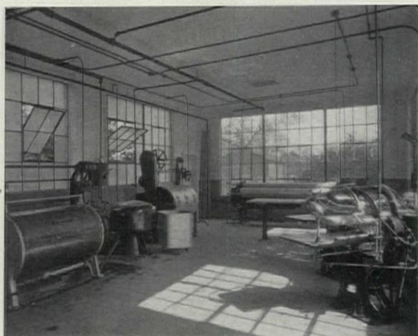
A Well Equipped Hospital Laundry
