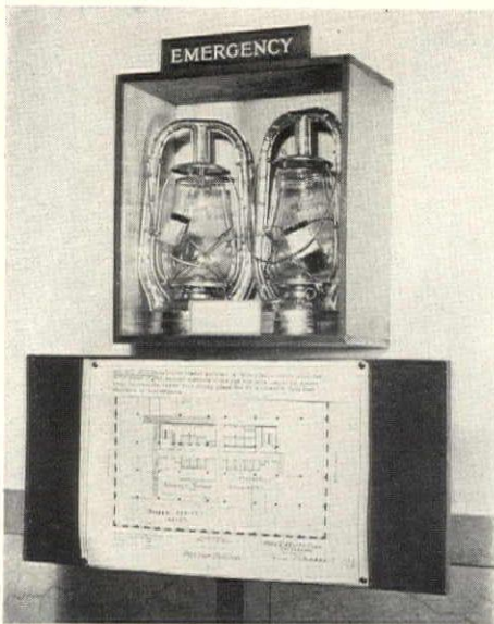
Lanterns in glass front cabinets supplement emergency lighting in event of power failure, are placed in all refuge areas. Below is plan of area considered safe.
