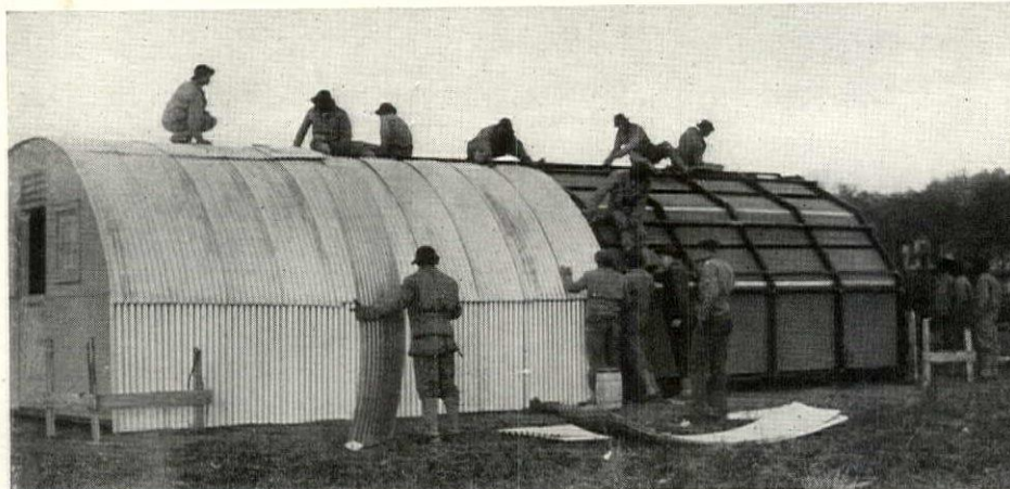
ARMY HOUSING tries its hand at prefabrication and creative design: (above) A test structure at Fort Belvoir, highly favored by military authorities since its knocked-down compactly shipped plywood panels simplify work in the field. Developed by National Housing Co.'s John Allen Boyle. (below) An improved type of troop shelter, the "hutment." Chief advantage over tents: earth can be banked along sides as protection against shrapnel. To convert tents into hutments in the Army's 24 tent camps will cost an estimated $25 millions.
