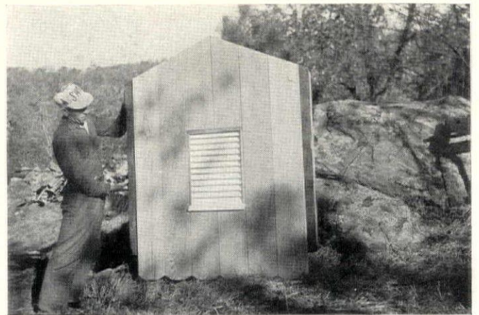
Ridge ventilator consists of louvre slats rabbeted into studs at sides, requires no frame and but little trim.
