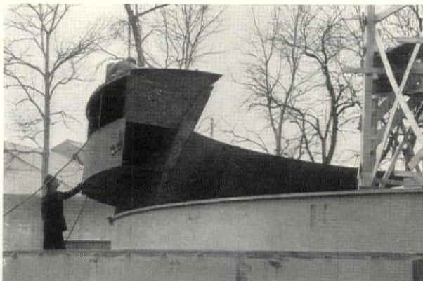
Air conditioning is distributed through a single, ring-shaped duct of welded steel, which acts as a retainer for the main dome and stiffens the entire structure. Duct is of welded steel, hung from steel angles.
