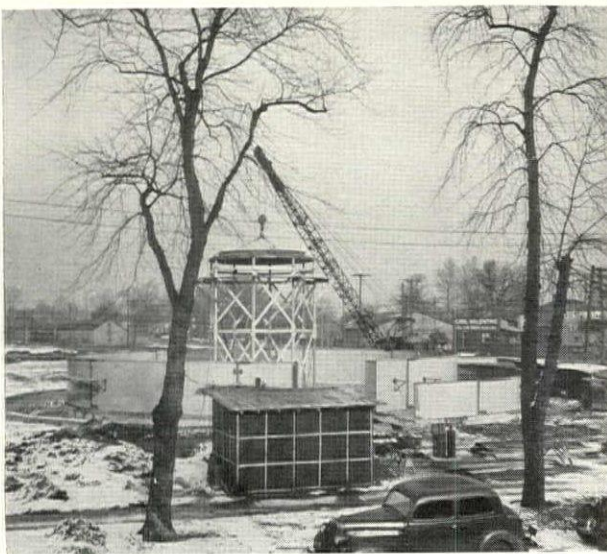
2 First stage in erection shows vertical wall plates in place and scaffolding supporting middle section of central dome; crane used to position sections.
