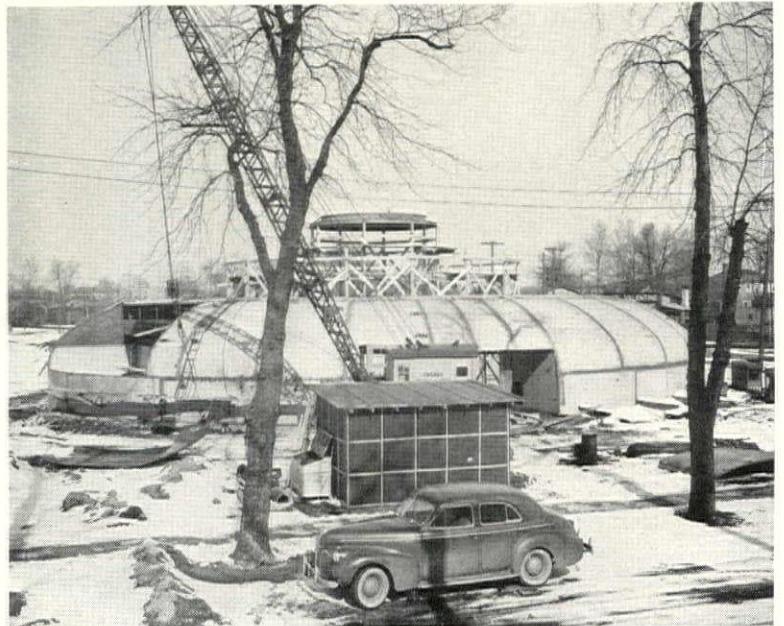
5 Lean-to roof almost complete. In left foreground, note curved roof section which derrick is about to lift into place.
