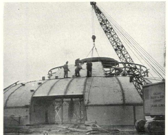
6 Main dome was completed last, by joining two rings of curved plates above the juncture of the lean-to roof with central section on scaffolding.
