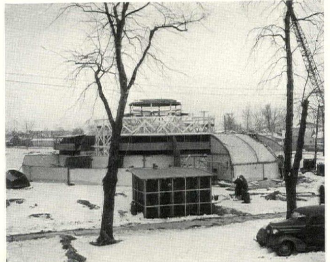
4 General view at same stage as 3, shows portion of outer "lean-to" roof in place, radial steel partitions, and (left) sectional view of first unit of inner dome and duct.
