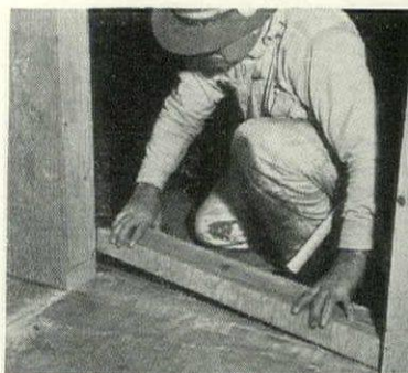
PANELS are shipped with a small integral strip across bottoms of door openings. This is sawed free after walls have been erected.
