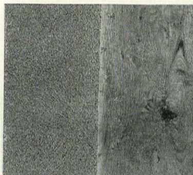
PLASTIC PAINT applied in two coats covers knot-holes and defects; provides a durable, smooth interior finish.
