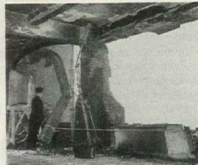
Only a few steel beams were damaged; plants on the window-sill of an adjoining office were unharmed.
