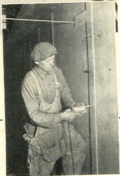
BOTTOM: Mechanic sinks holes in asbestos-cement batten which is securely bolted to Cemesto wall unit at joints.
