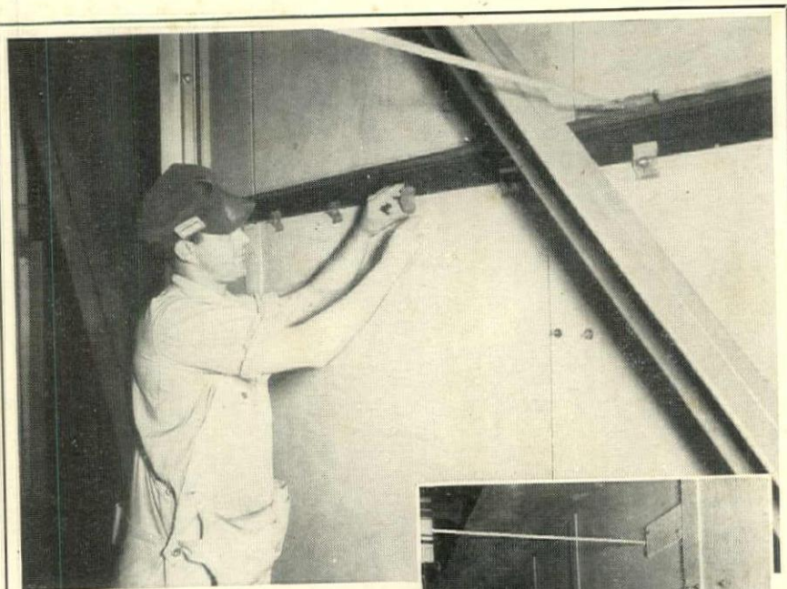
TOP: Workman demonstrates application of Cemesto wall unit at recent Cadillac Motor Car Co. factory addition, Detroit, Mich. Cemesto is rigidly held in place on steel beams by means of easily-applied metal clips.
