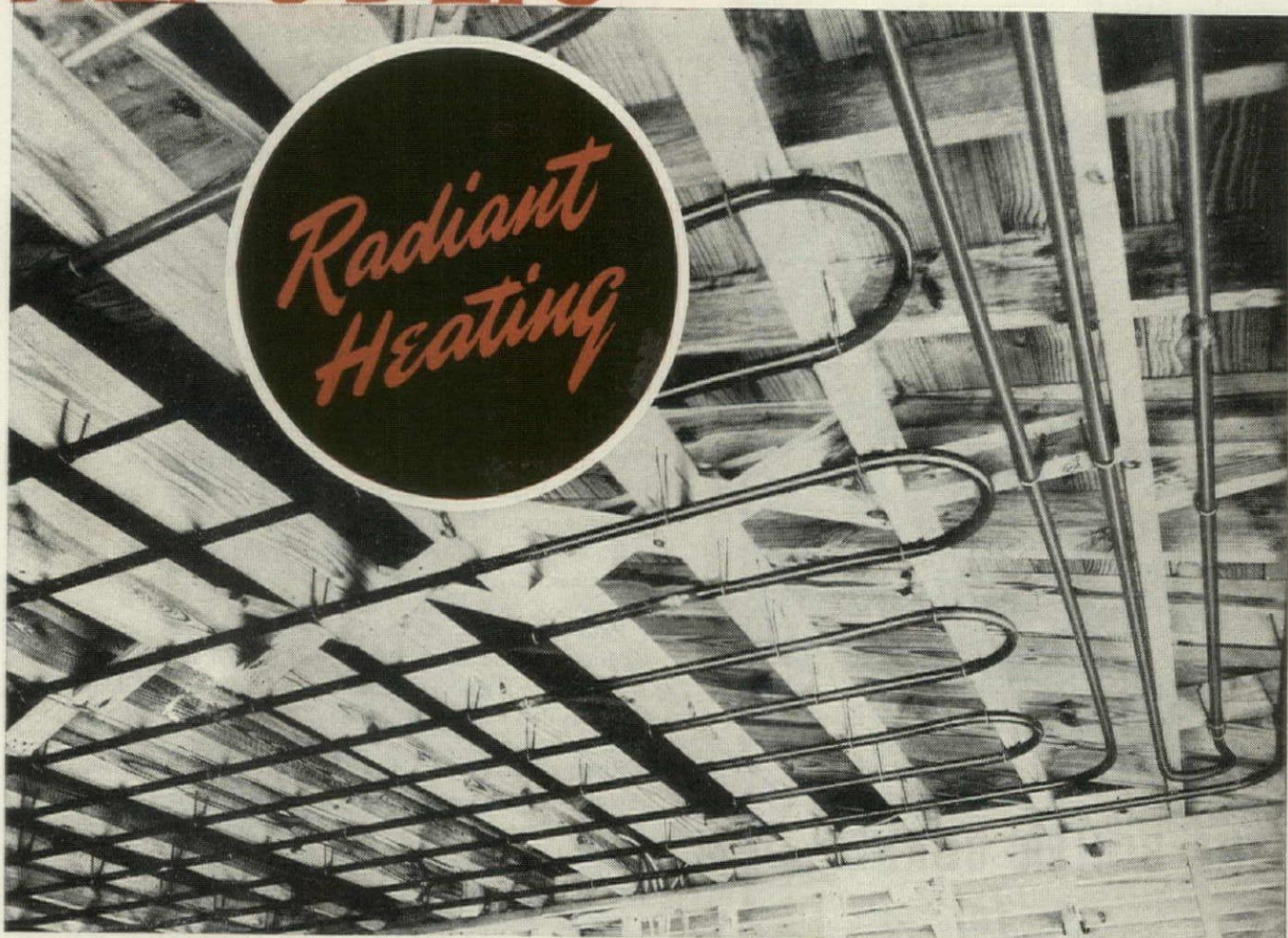
The superior bending qualities of Republic Pipe make a big difference in jobs like this where 207 bends are required in installing 2500 feet of \frac{3}{4} " pipe for radiant heating.
