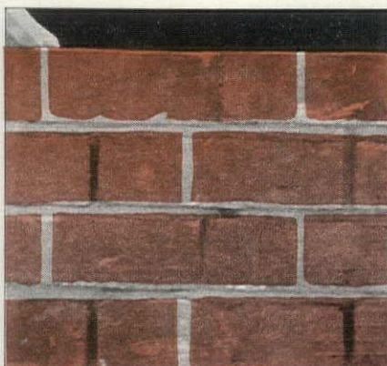
This encourages the bricklayer to fill the head joints, since proper tooling cannot be done if mortar is lacking.
