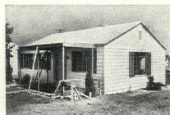
Porch being applied to the completed house, showing Reynolds Lifetime Aluminum Clapboard Siding with its final (second) coat of paint.
