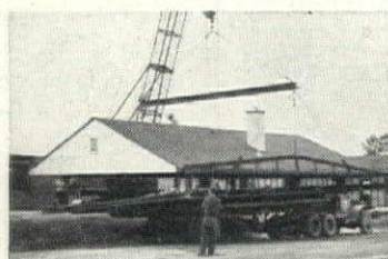
Loading complete roof on special truck. Reynolds Lifetime Aluminum Weatherboard Siding on gable end. Louvre also of Reynolds Aluminum.
