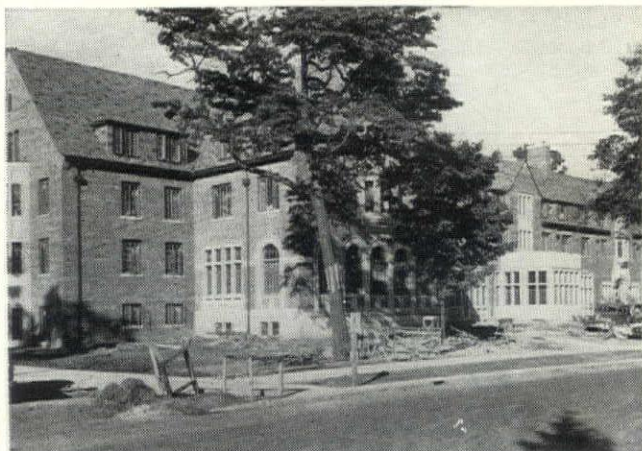
Ridges, flashing, valleys and gutters of Revere Copper protect 5 new dormitories at MICHIGAN STATE. Architect for Girls' Dormitories: Ralph R. Calder, Detroit; Contractor: Christman Co., Lansing. Architect for Men's Dormitories: Orlie J. Munson, Lansing, Contractor: Reniger Construction Co., Lansing. Sheet Metal Contractor: Michigan Sheet Metal Works, Lansing.
