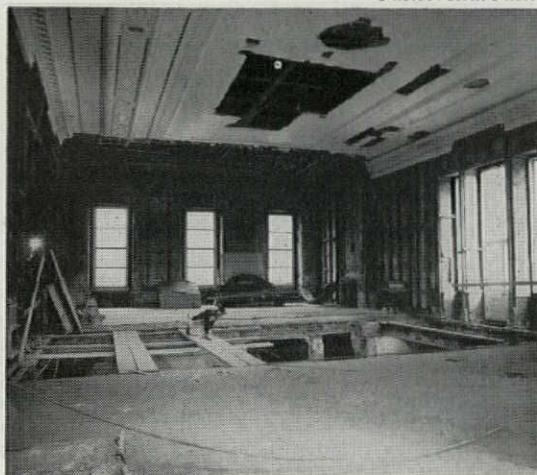
INADEQUATELY FRAMED span of East room on first floor will get new brace with steel construction.
