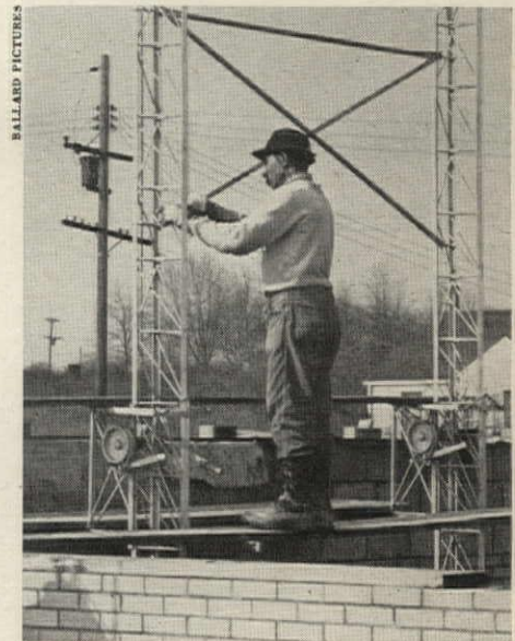
PRODUCTIVITY BOOSTER for mason is this adjustable scaffold. It keeps mason at optimum working position, increases his productivity by 20% to 25%. Three such scaffolds are on market now.
