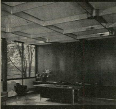
This executive office in the Research Administration Building, one of seven at the General Motors Technical Center air conditioned by Thermotank, shows a typical installation of Thermotank's custom-designed diffusers with integrated sprinkler heads
