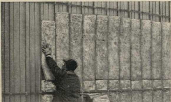
Noncombustible insulation is inserted between the back-up panel and the steel bars.
