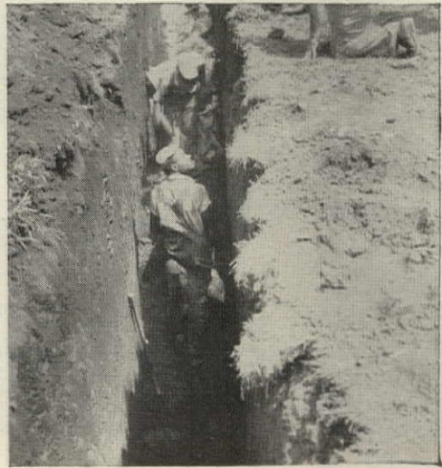
ONLY 5 MEN (unskilled) were needed to do the job: two in the trench and 3 above.
