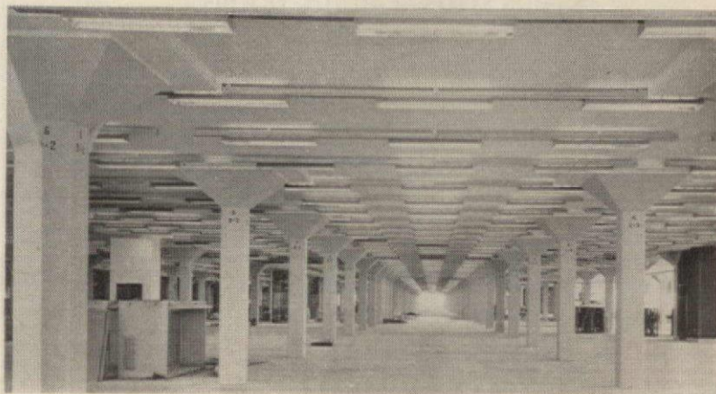
Huge record-storage area, especially arranged for vertical lighting of files with Day-Brite fixtures.
