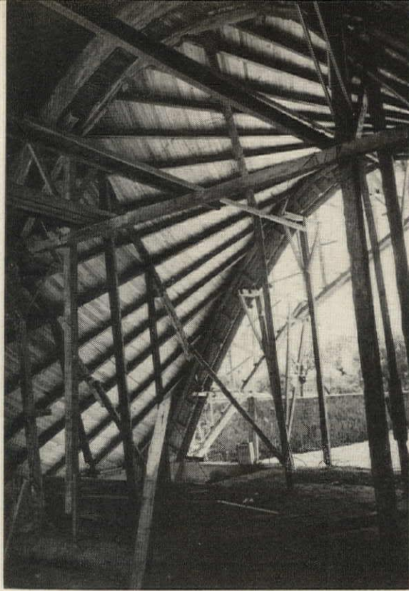
Formwork for one of the masterly shells by Architect Felix Candela in Mexico illustrates complex wood construction ironically required for bold exploitation of reinforced concrete's plasticity.
