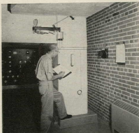
Primary air supply regulated by Sub-master Thermostat and Powerstroke damper motor.
