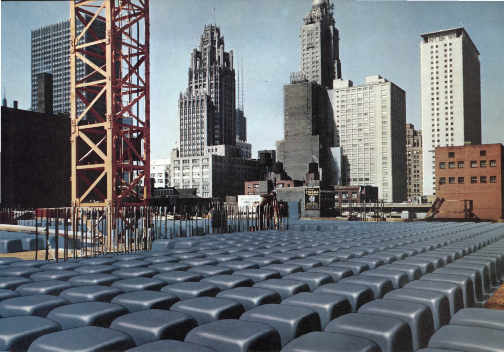
Time & Life Building, Chicago, Illinois 600,000 sq ft of Ceco Steeldome services Harry Weese & Associates, architects-engineers James Rudeman, structural engineer Turner Construction Company, contractor
