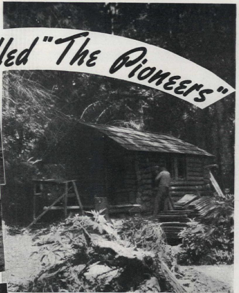
Finishing touches on the small cabin at the edge of the forest
