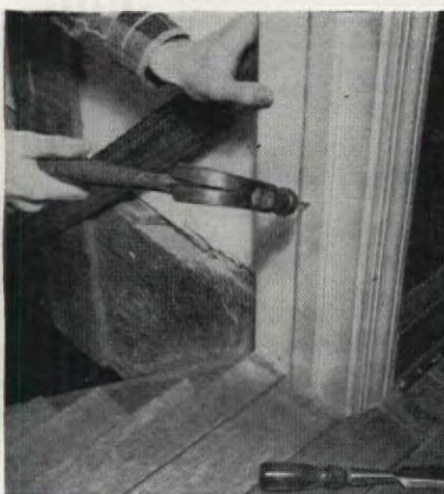
8. If the door sticks against the stop, carefully pry up stop with a chisel and reset it slightly away from the door to provide additional clearance
