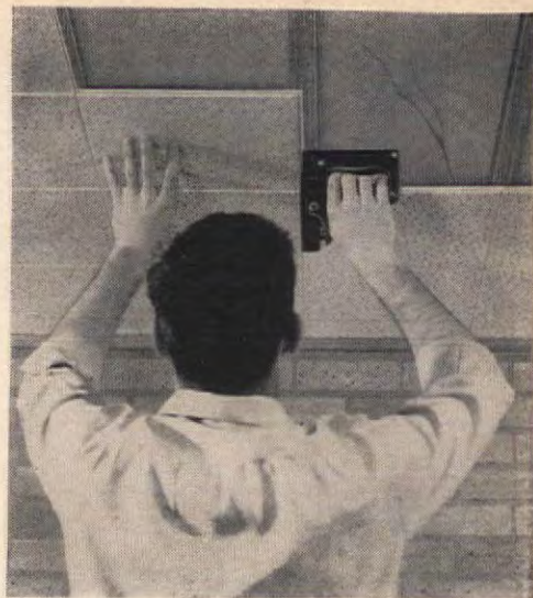
Mr. Irvin put up his ceiling of Armstrong Cushiontone in a single week end. The job went much faster than expected because he found the 12" x 12" tiles were so easy to apply. Actually two jobs were done at once. Besides providing much needed quiet, ugly cracks were covered permanently and without the mess of plaster.
