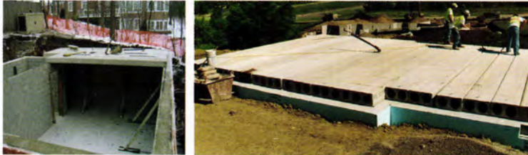
Photos of Molin Concrete hollow core planking being installed on a home
