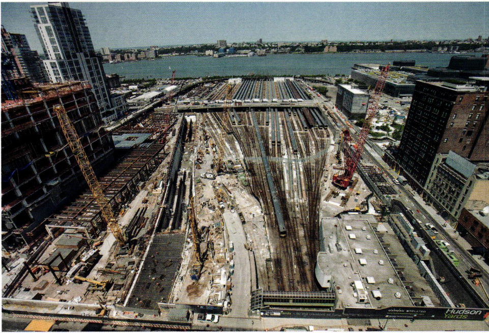
Top: A view of Hudson Yards in 2014, as giant cranes and boring machines constructed a platform that today supports office towers, apartments, and a shopping center. A concrete casing as route protection for Amtrak's future trans-Hudson tunnel was simultaneously constructed.
