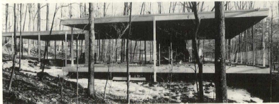
Under construction in Bethesda, Md., this residence for Dr. and Mrs. Harry Galblum is framed in light steel structural members. Architect, Harold Lionel Esten.
