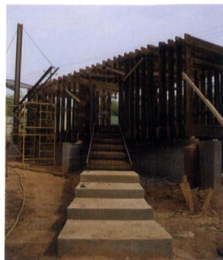
A view of the Memorial Block as the major structure is reaching completion. Reclaimed wood from the Keese Barn forms the ribs.
